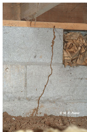
Fig. 6: Telltale signs of termites: mud tunnels
