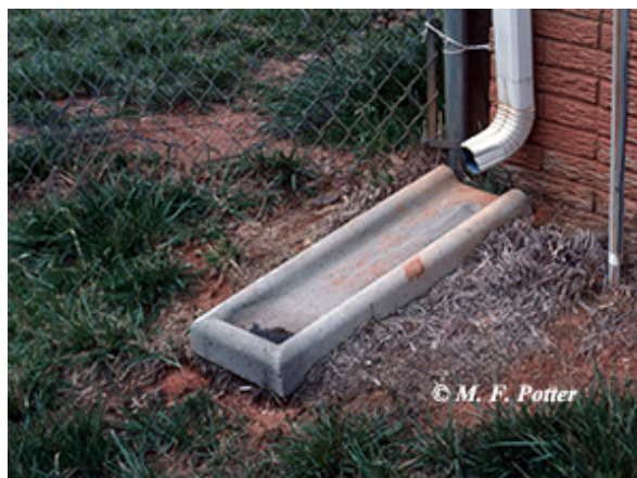
Fig. 2: Divert water away from foundations. Downspout splash blocks are helpful, but this one is facing in the wrong direction.
