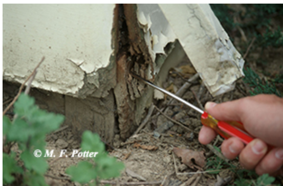
Fig. 1: Wood-to-ground contact aids entry into buildings.
