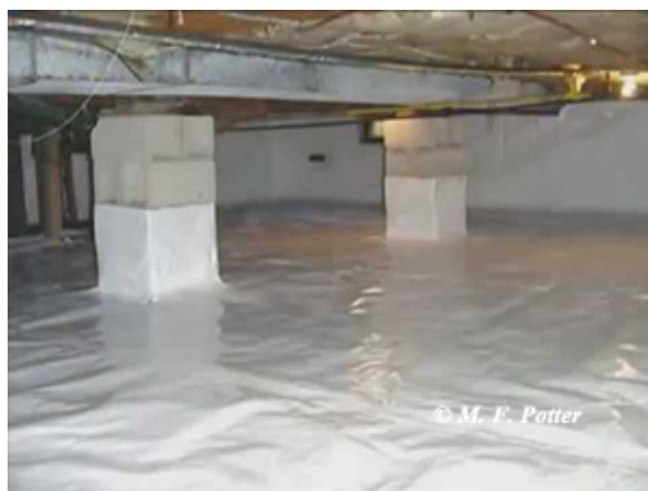
Fig. 3: Moisture in crawl spaces can be reduced by installing plastic sheeting.
